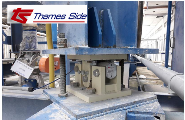
PVC & CaCO 3 , Silos weight monitoring system
